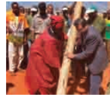
IFAW HELPED TAVETA AREA COMMUNITY MEMBERS AND THE KENYA WILDLIFE SERVICE START CONSTRUCTION OF A 78-KM ELECTRIC FENCE NEAR TSAVO NATIONAL PARK TO REDUCE HUMAN-ELEPHANT CONFLICT. DR. NAOMI SHABAN, TAVETA PARLIAMENT MEMBER, AND IFAW BOARD MEMBER DR. MANILAL CHANDARIA RAISE A FENCE POLE.
